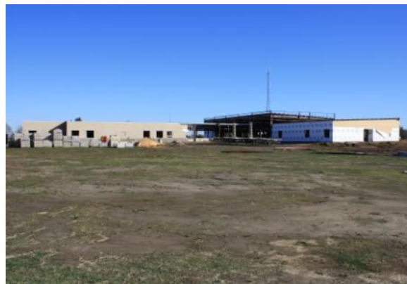
Construction of the new Nursing and Allied Health building on the ANC Blytheville main campus is well underway, with anticipated completion in 2012.
